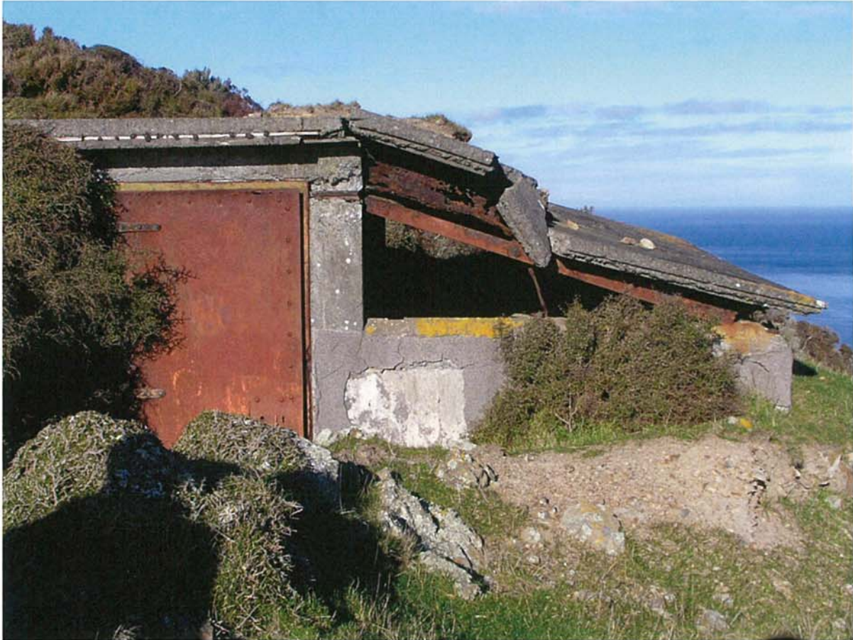
Observation bunkers in need of stabilising before the public can access the site
