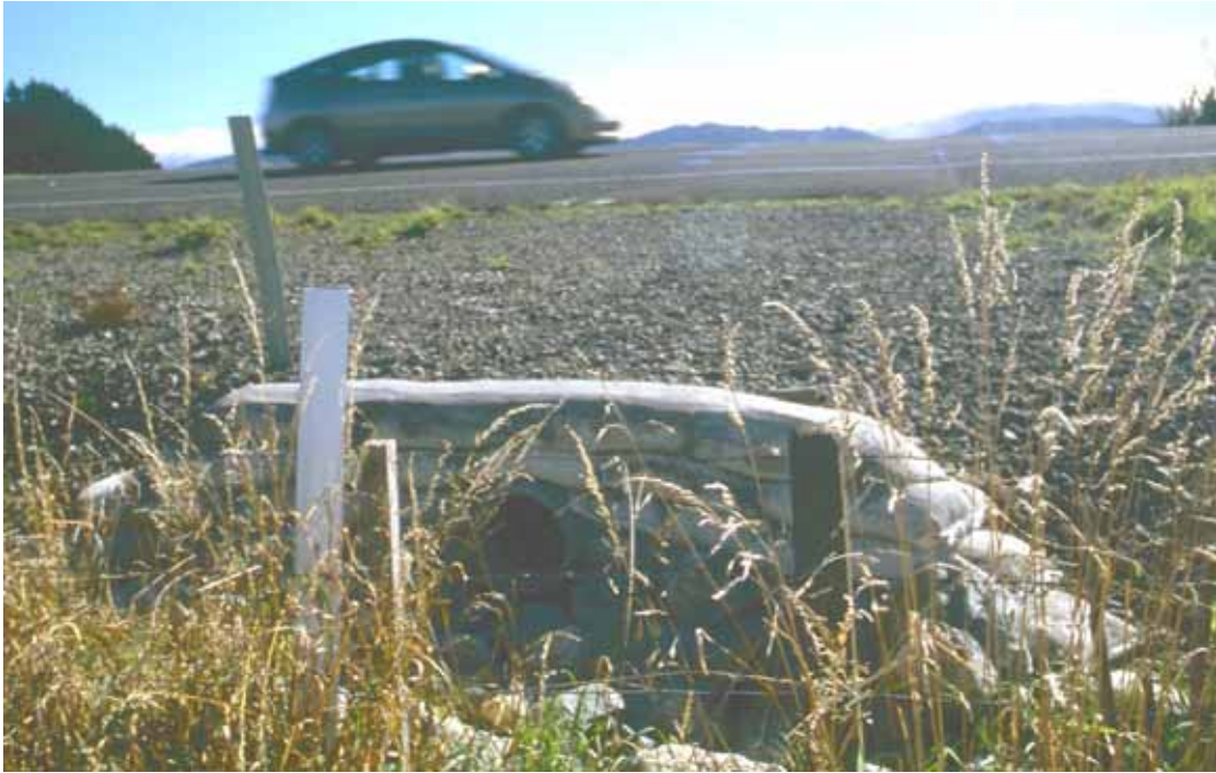
Photo 5.8.5: Metalled shoulder of State Highway 2 channelling road runoff through culvert to wetland.
