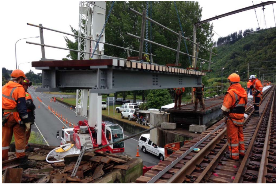
KiwiRail contractors lower a new low profile bridge span on to Bridge 30 at Silverstream
