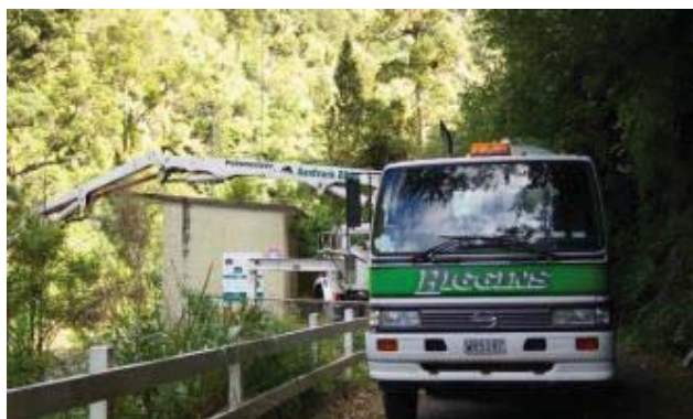
Maintenance activities at Kaitoke Weir. The threat of contamination from vehicles entering the water collection areas is actively managed via means such as standard operating procedures and works contract conditions
