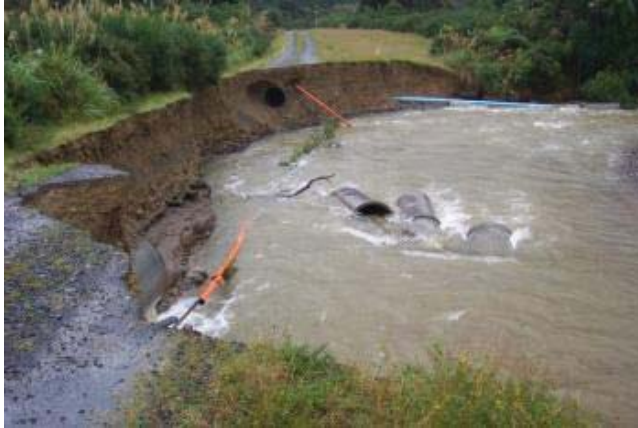
A storm in the Wainuiomata catchment downstream of the intake in 2005 caused heavy erosion of an access road and broke water supply pipe and power cable.
