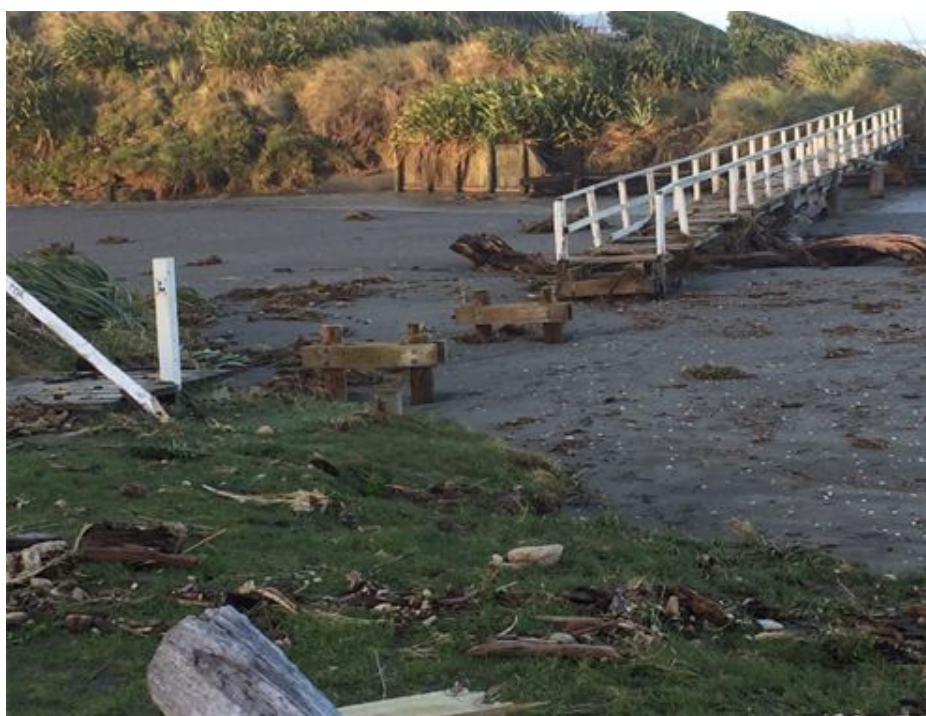
Storm damage after ex Cyclone Gita at the Wainui Stream mouth, Queen Elizabeth Park, February 2018. For visitor safety the remaining sections of the bridge were removed.
