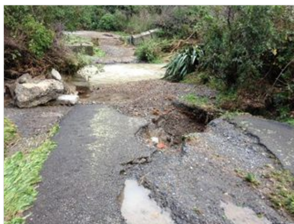
Climate change is already presenting challenges for park management. In 2015 the Korokoro stream catchment in Belmont received very high rainfall in a short period which resulted in flooding that damaged many of the assets in the valley.
