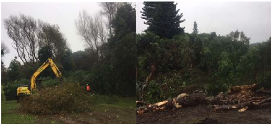
Contractors removing numerous old and hazardous Poplars alongside the lower Wainui Stream in Queen Elizabeth Park
