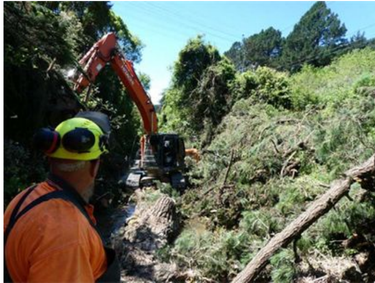
Porirua Stream Blockage
