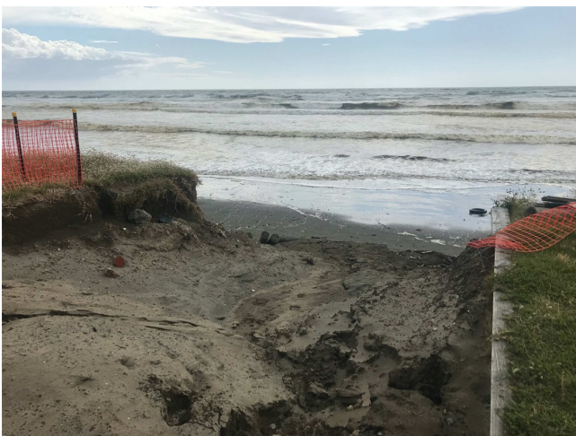
Figure 19 - Collapsed ramp, club side
