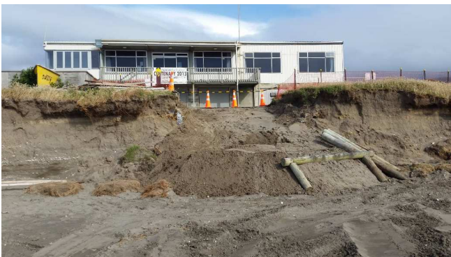
Figure 18 - Collapsed boat ramp, oceanside
