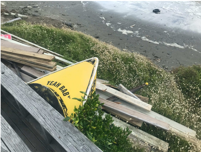
Figure 17 - Collapsing dunes underneath the patrol tower
