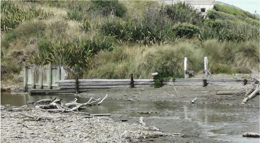
Figure 6: Wooden sea walls placed historically to limit stream break-out and erosion on the southern side of the stream entrance.
