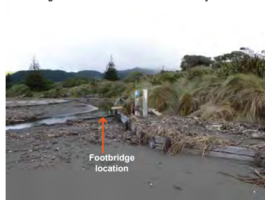
Footbridge across Wainui Stream washed away
