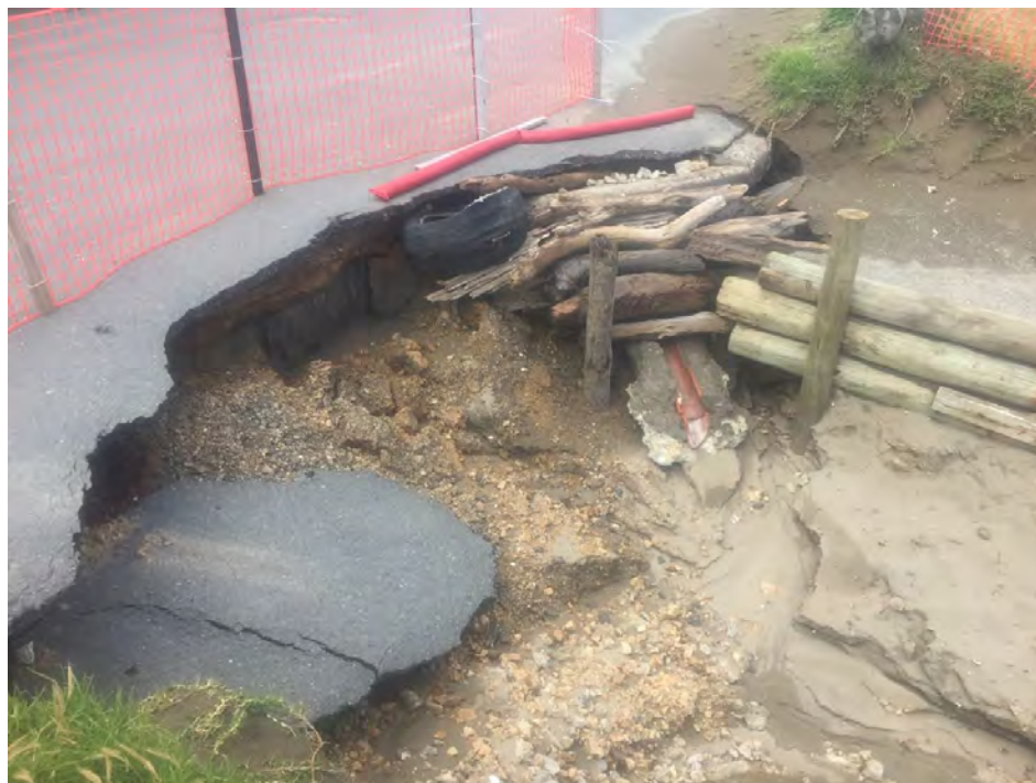
Plate 1: Erosion undermining the beach front vehicle access road at the surf lifesaving club. 19 November 2020.
