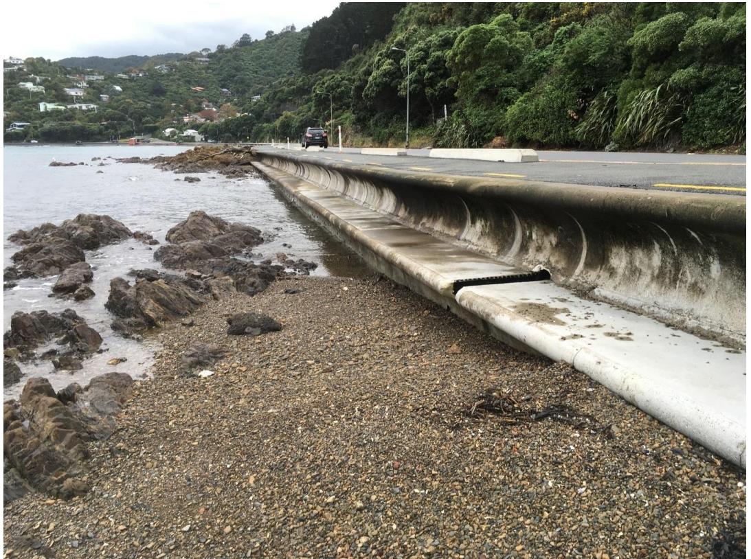
Figure 10: Recently constructed double curved seawall at southern York Bay with sediment accumulation and hence transport in the coastal zone at the foot of the seawalls.
