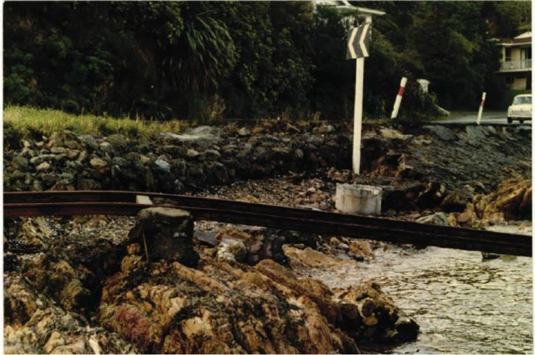
Figure 3: Erosion and undermining erosion of wire and stone wall at northern end of Lowry Bay (Jan 1991). [Source: HCC archives].
