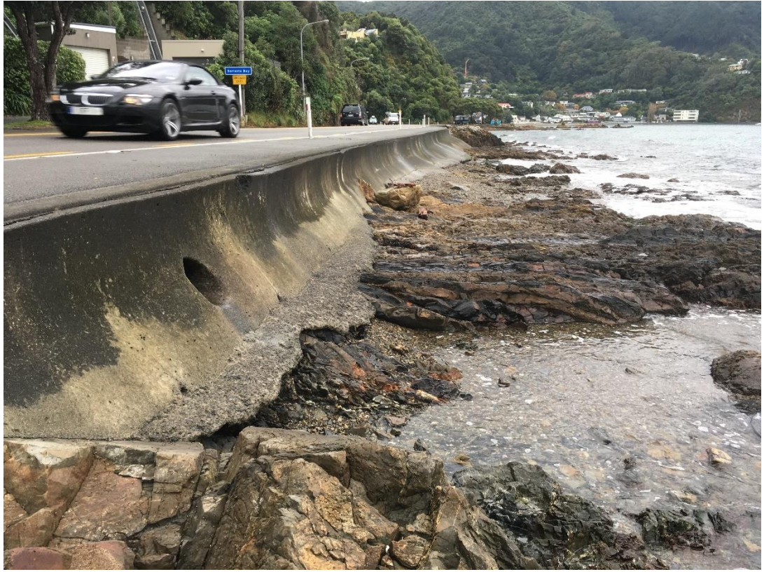
Figure 4: Erosion and undermining of seawalls repaired with concrete along rock platform between Pt Howard Bay and Sorrento Bay (May 2017). [Source: M. Allis (NIWA)].
